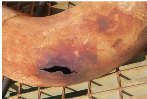
Figure 2(Typical Shear on the Elbow)
