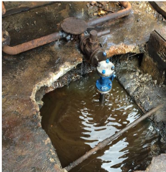
Figure 8.0 (2-inch Ball valve closed and blinded)
