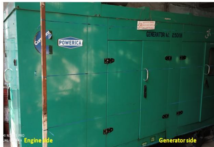
Fig 1. DGSet (with enclosure doors closed)
