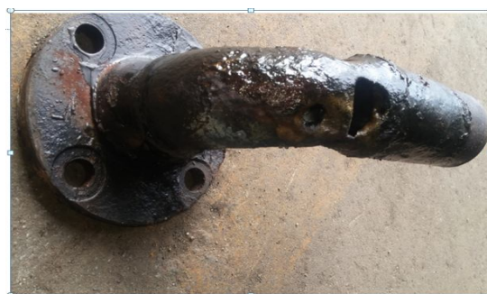
Figure 12.0 (Ruptured Elbow Eliminated)
